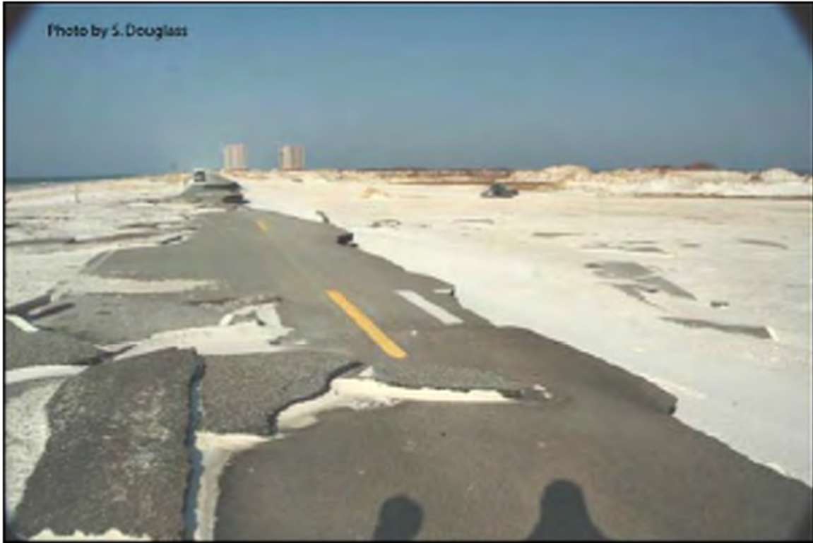
Figure 8.3. Example of pavement damaged by Hurricane Ivan. (photo looking west on Florida 399, J. Earle Bowden Way, Gulf Islands National Seashore, September 2005)
