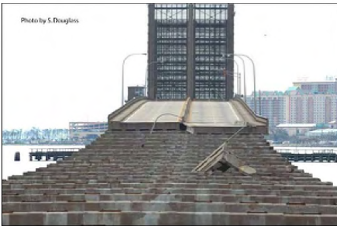
Figure 9.14. US 90 bridge over Biloxi Bay, Mississippi showing the spans at higher elevations were not removed (photo looking southwest from Ocean Springs 2/19/06.)
