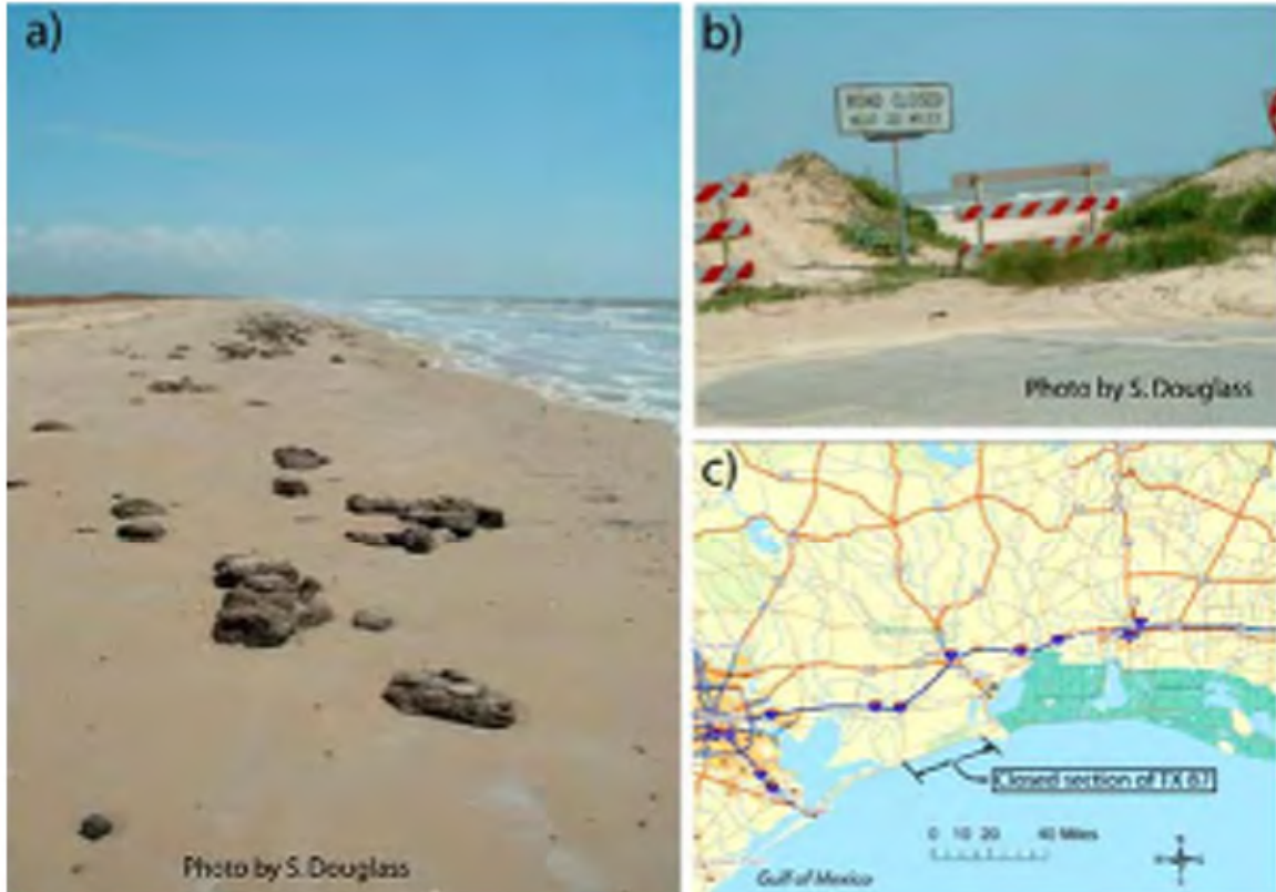
Figure 7.5. Road destroyed by shoreline recession: a) broken pavement on the beach at the old location; b) south end of the closed section; c) location map. Texas Highway 87, Jefferson County (2002)
