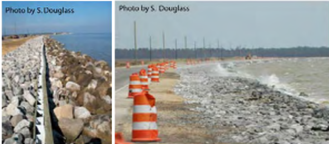
Figure 6.15. A revetment with rocks too small to withstand wave attack
