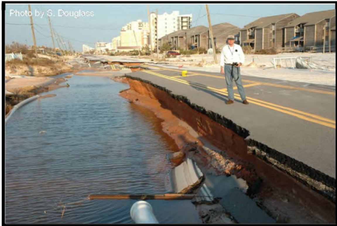
Figure 8.2. Example of pavement damage due to storm surge. Florida 292 on Perdido Key, Florida after Hurricane Ivan (Sept. 2004)
