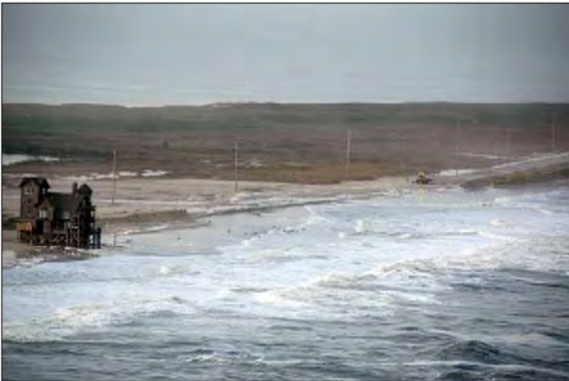
Figure 8.1. A coastal road being overwashed during a storm. North Carolina Highway 12, November 23, 2006 (North Carolina DOT photo)
