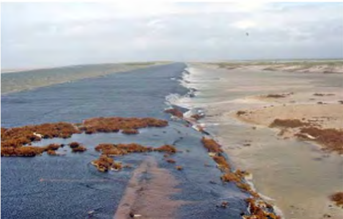
Figure 8.8. Weir-flow damage occurring. (Florida 399, Fort Pickens Road, Gulf Islands National Seashore; July 2005; FHWA photo).
