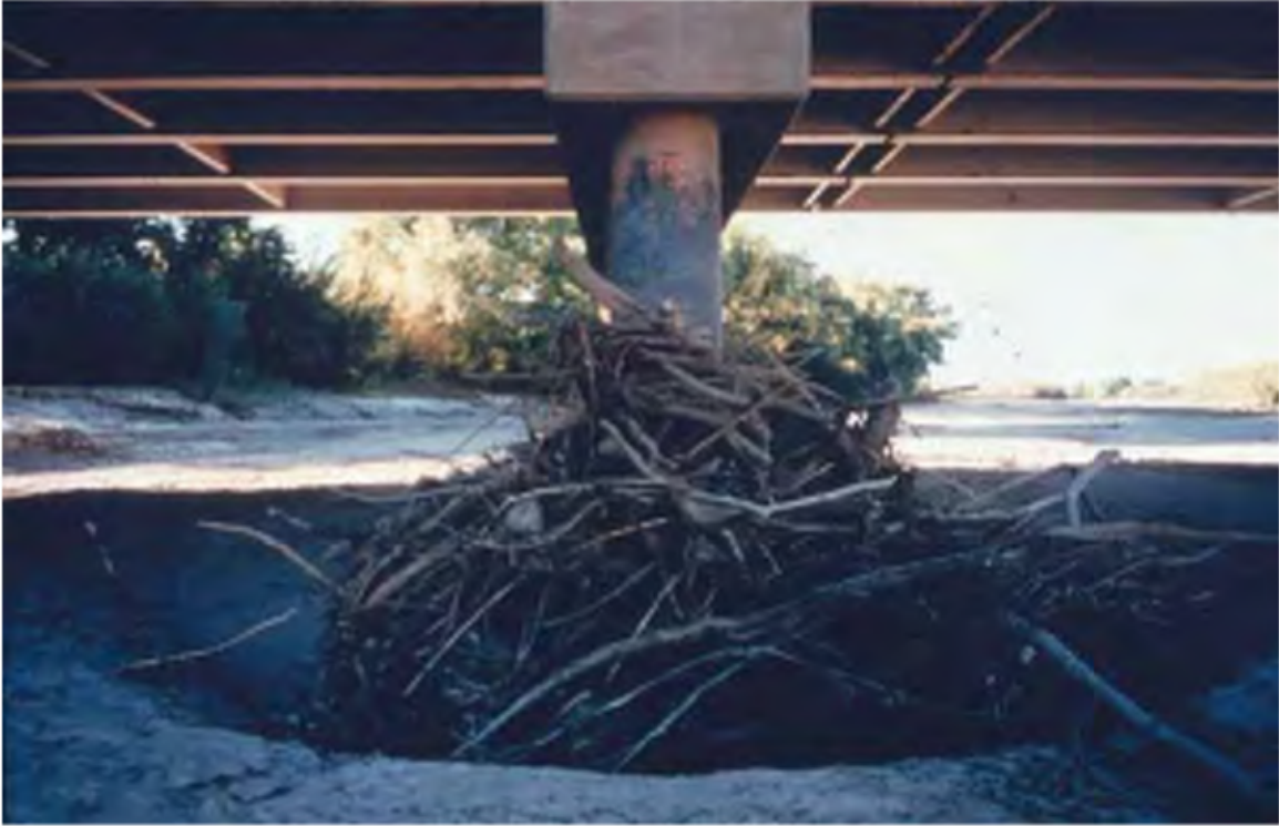
Figure 9.5. Scour at a Coastal Bridge Pier
